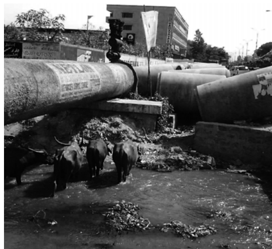
Fig. 1 Photograph shows the sewage water pipeline is one of the potential hazards causing H. pylori transmission in India. The pipeline is leaking near the gutter and the buffalos are grazing in it. This is a common picture in most of the cities in India presenting the view of water contamination and transmission of water-borne diseases.
